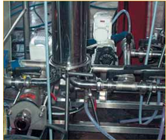
Pump on filtering pallet (wine production)
