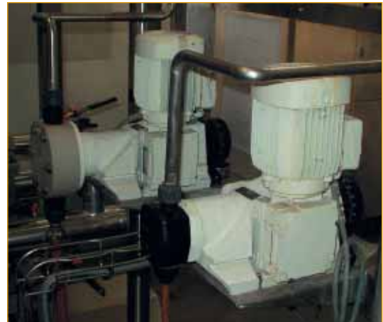
Metering of soda and acid
