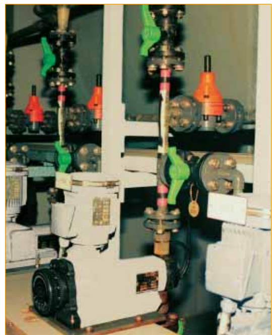
Ferric chloride pumping in purification station
